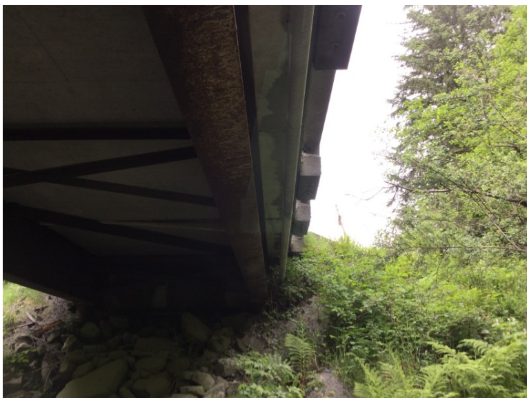
Utilities on downstream end
